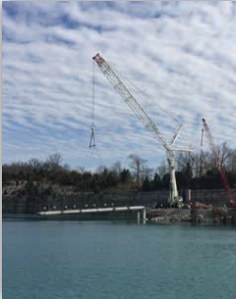
Dave O'Mara and Sterett Crane working on the new water intake system in North Vernon
