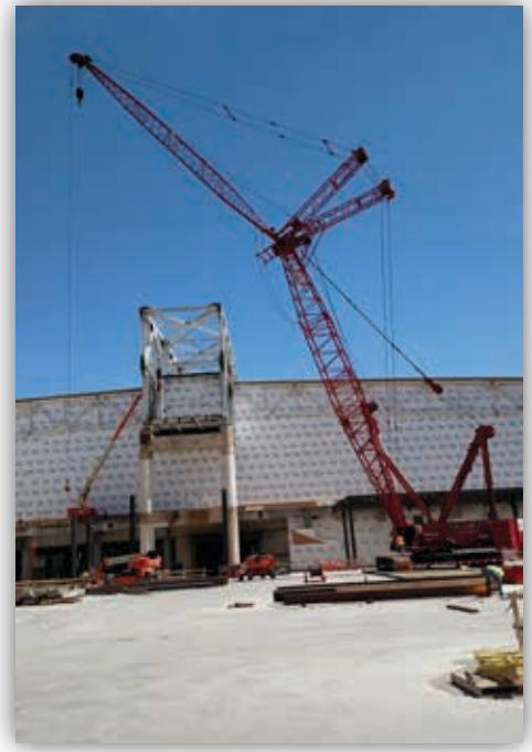
Midwest Steel working on Kentucky International Convention Center in Jefferson County, KY
