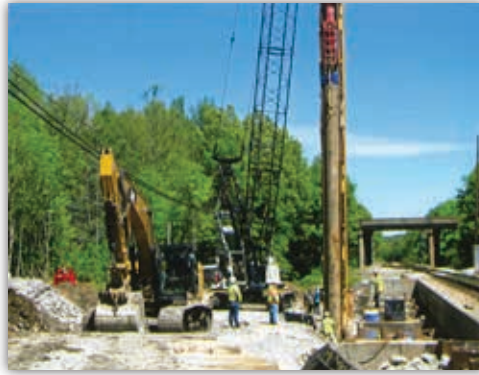
Ragle, Inc. at the CSX Railroad Bridge project in Hopkins County, Kentucky.
